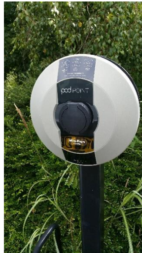
36 – Pod point charger
